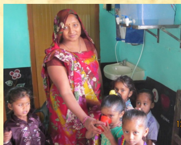
Newly Installed RO unit at the Aanganwadi of Pilupura village in Sanand
